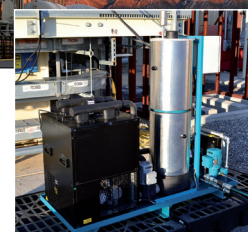
CJC™ Varnish removal Unit VRU 27/108 PV installed
